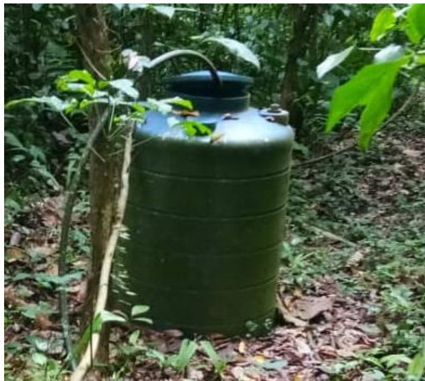
Figure 2: Main water tank.
